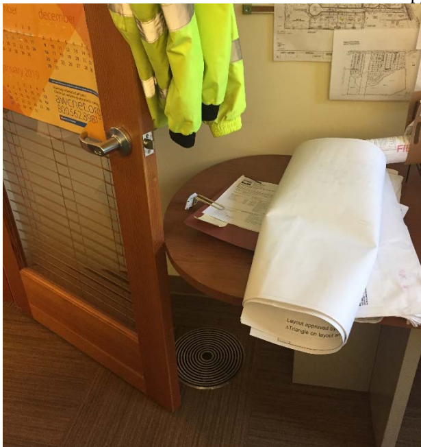
Office door does not fully open.
