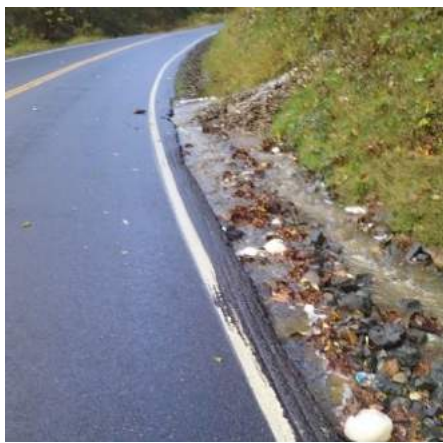
Stormwater runoff on the side of Jovita Boulevard in Edgewood transports pollutants and can damage the roadway.
