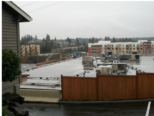
Figure 57 – Example of what NOT to do – unshielded equipment can be unsightly from adjacent properties.
