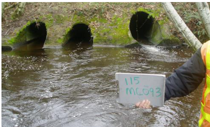
Before at Coffee Creek: culverts were barriers to fish due to high water velocities and insufficient water depth.
